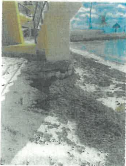
Looking East Note erosion
