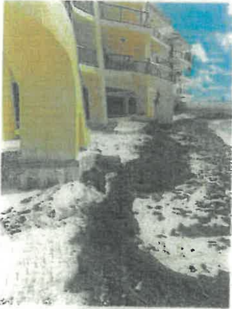
Looking East Note erosion
