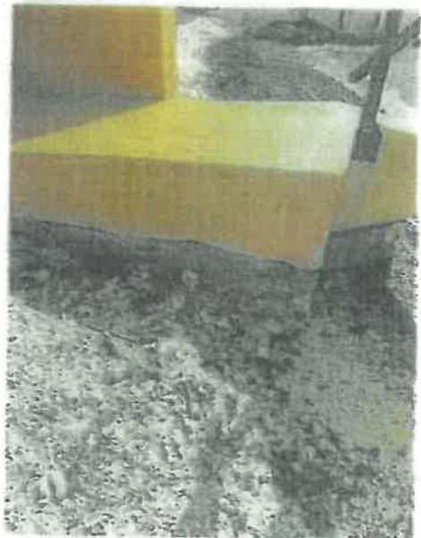
Looking East Note undermining
