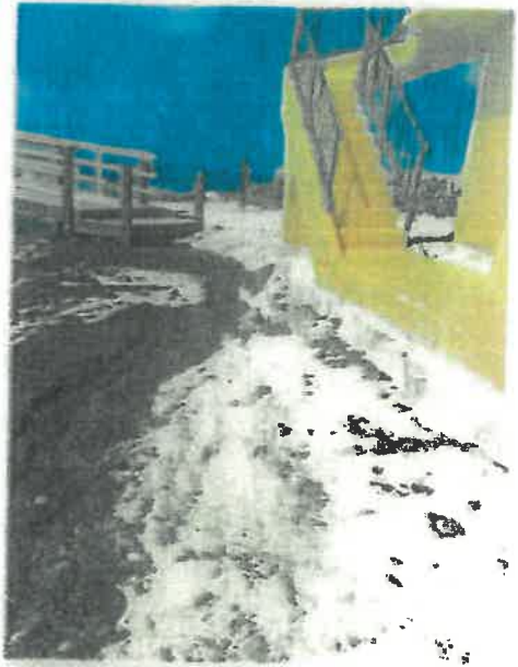
Looking West Note undermining
