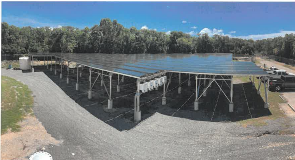
Picture of Key Largo Wastewater Solar Panels
